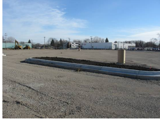
View from northwest portion of Property looking southeast across parking lot area
