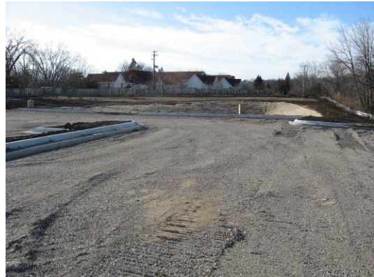
View from north-central portion of Property looking west at parking lot and storm-water pond
