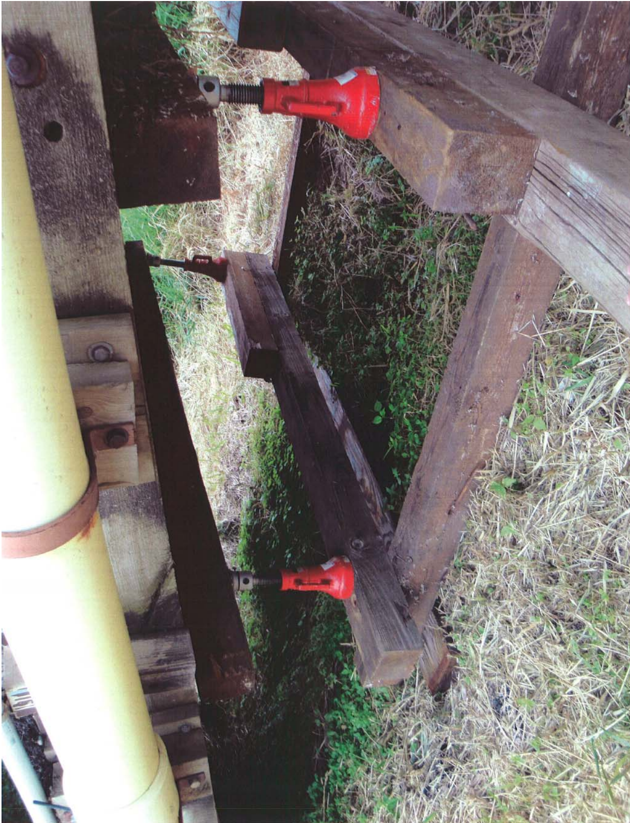
Photo 2: Jack to temporarily repair damage to trail bridge ramp
