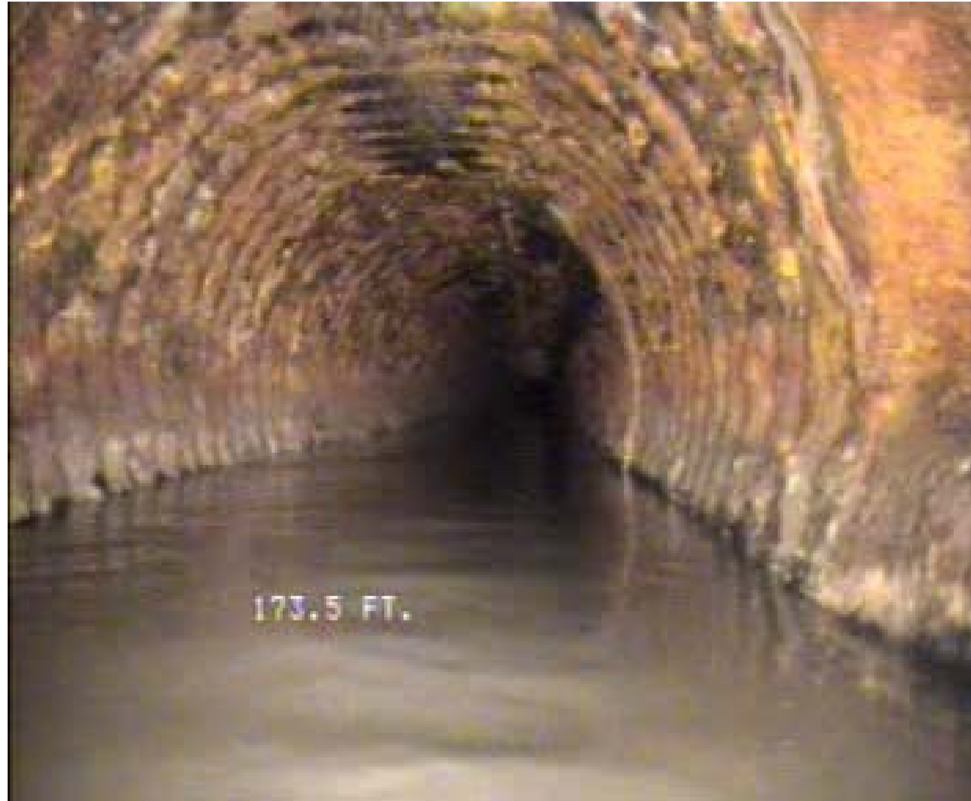
Photo: Corrosion damage to corrugated metal pipe
