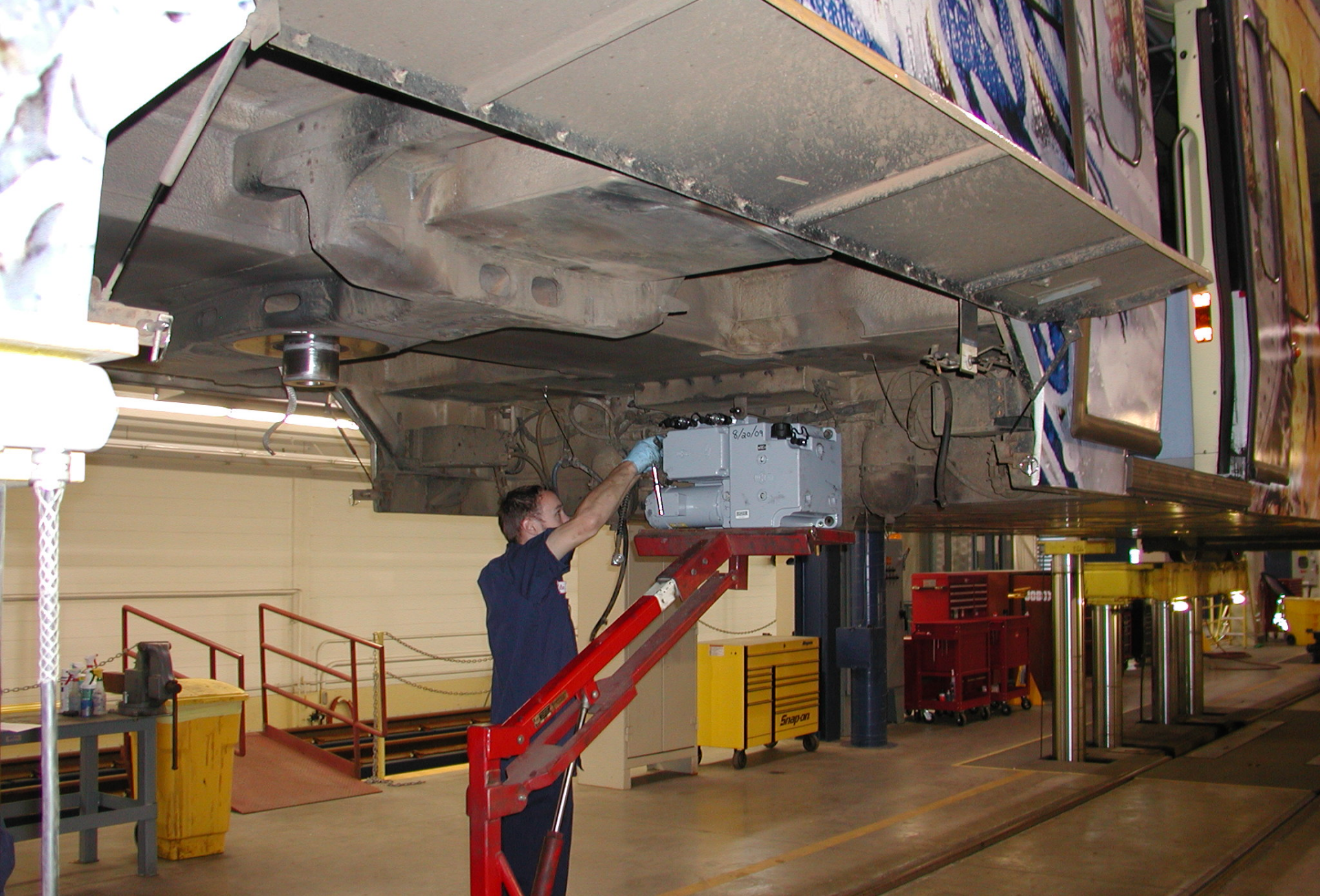
Power Truck has been removed and the rebuilt Electronic Hydraulic Control Unit is being installed
