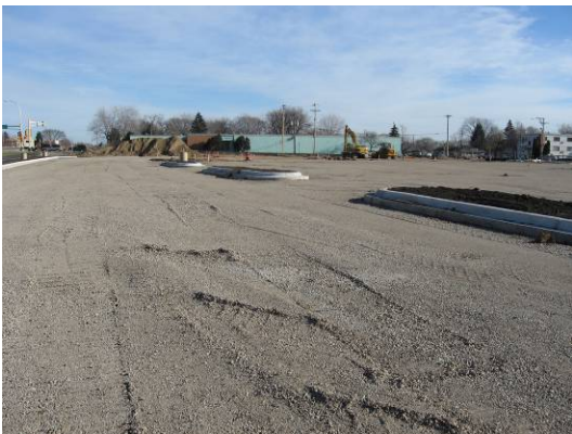
View from northwest portion of Property looking east across northern parking lot/driveway area
