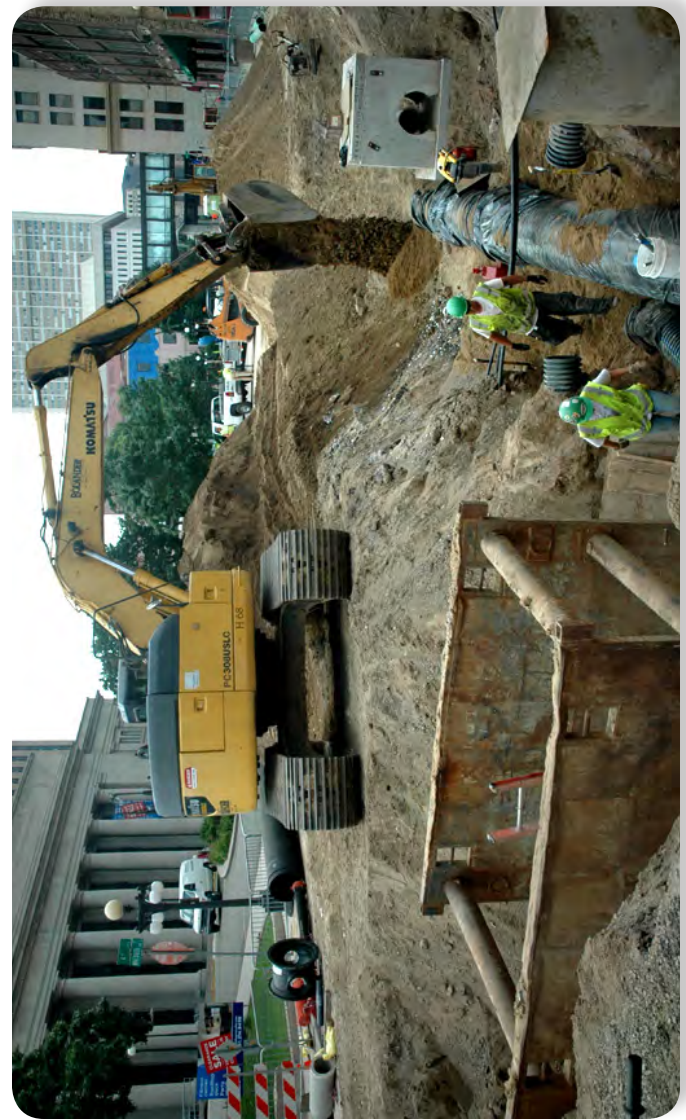
Figure 3-11: Early construction on the Central Corridor Light Rail, which is partially being funded using Federal New Starts
